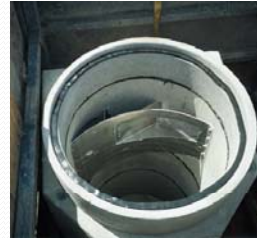
Hydrodynamic Separation Photo Credits: Contech Stormwater Solutions, Inc.
